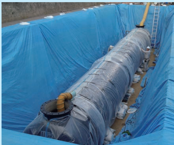
震災対策用飲料水貯水槽
