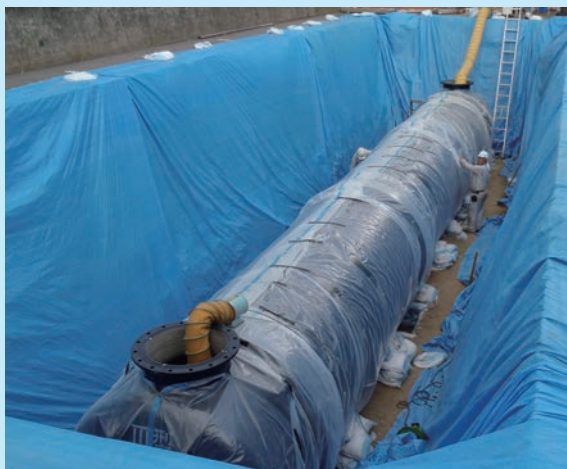
震災対策用飲料水貯水槽
